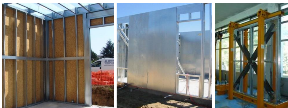
a) OSB panel sheathing-braced system b) Steel sheet sheathing-braced system [4] c) Strap-braced system
