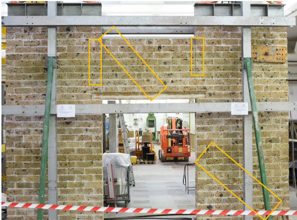
Figure 55. Crack pattern for intact URM, back side
