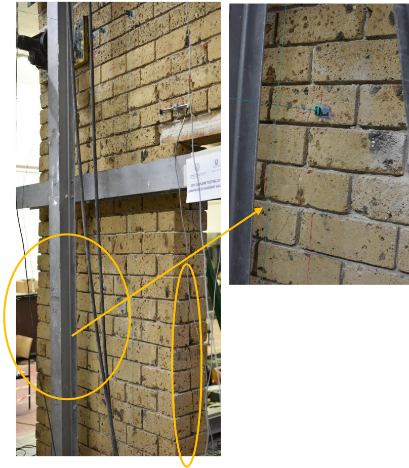
Figure 65. Crack pattern of loaded pier with details, deteriorated URM, frontal side.
