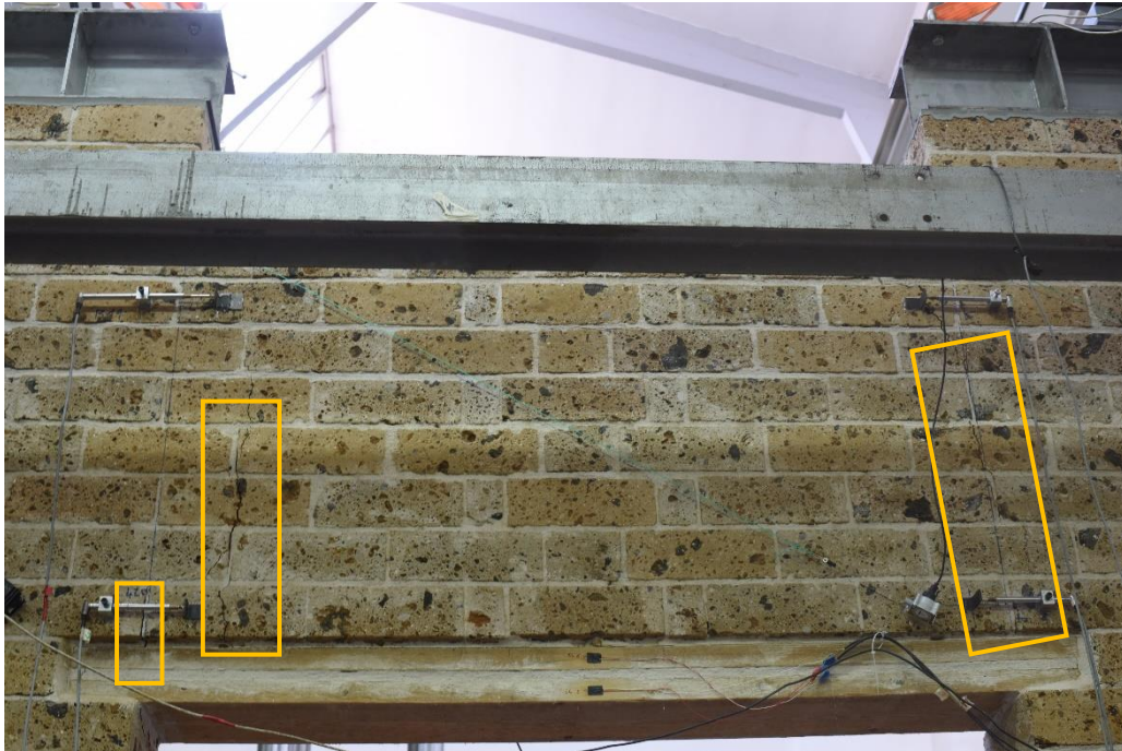
Figure 43. Crack pattern at 15mm of settlement applied to intact URM, frontal side
