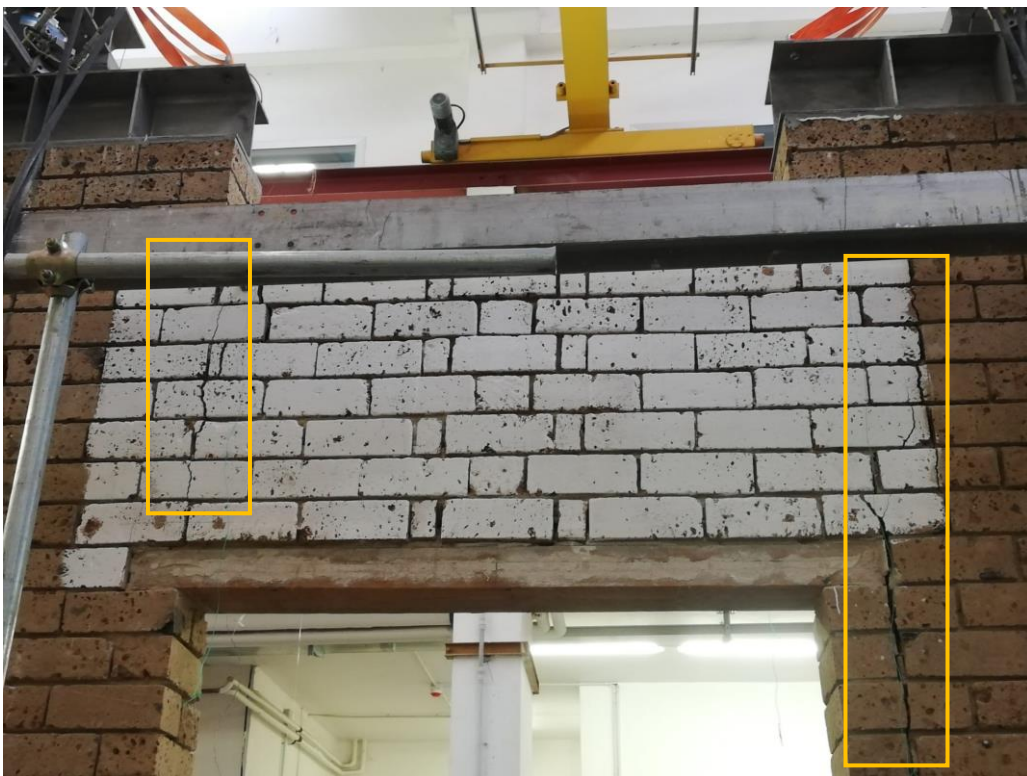
Figure 46. Crack pattern at 35mm of settlement applied to deteriorated URM, back side
