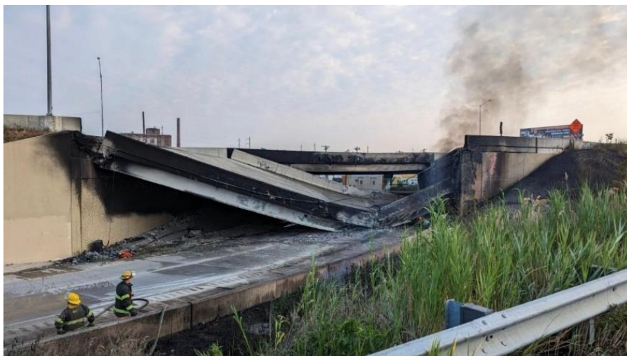
Figure 1.3. I95 collapse in Philadelphia after tanker fire, US, 2023 [6]
