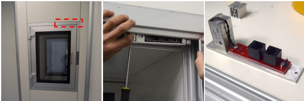
Figure 3.10: Damage of the electromagnetic lock of the inside door of pass-box, ID 110 test.
